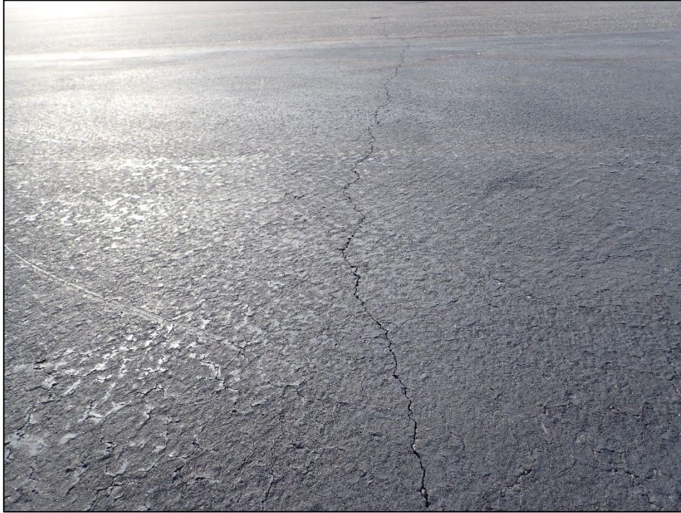
AP-01-09: L&T Cracking
