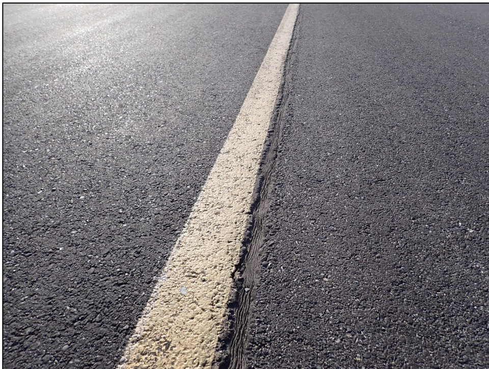
TW-01-13: L&T Cracking
