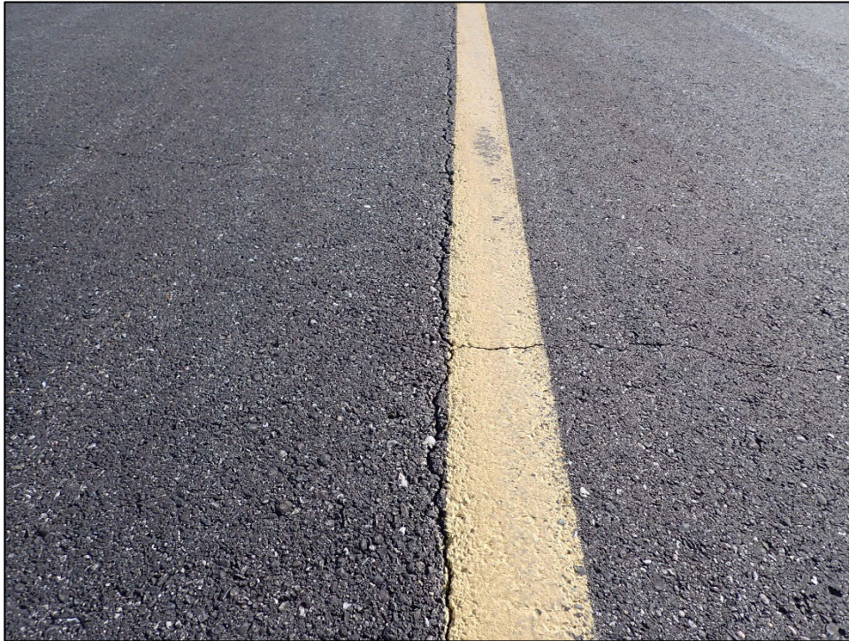
TW-01-12: L&T Cracking
