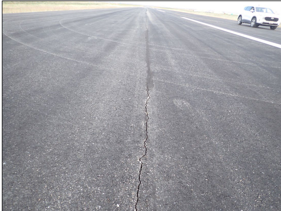
RW08-01-06: L&T Cracking
